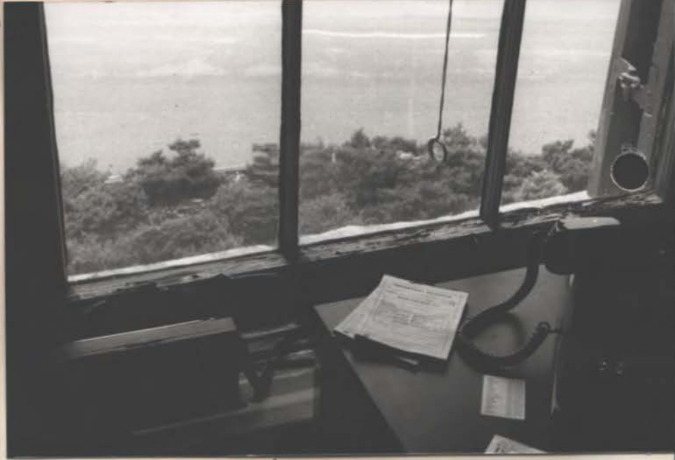
2ND FL. S.W. OFFICE ← Moist. damage to sash
