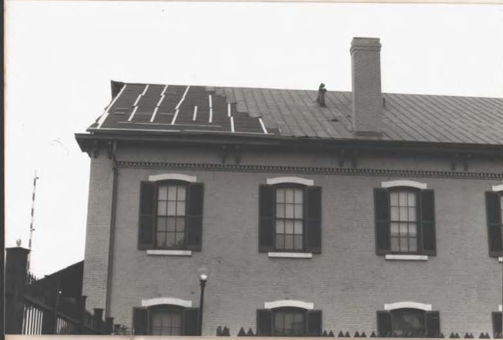
N ← ROOF PITCH SOUTH WALL ROOF DENTED
