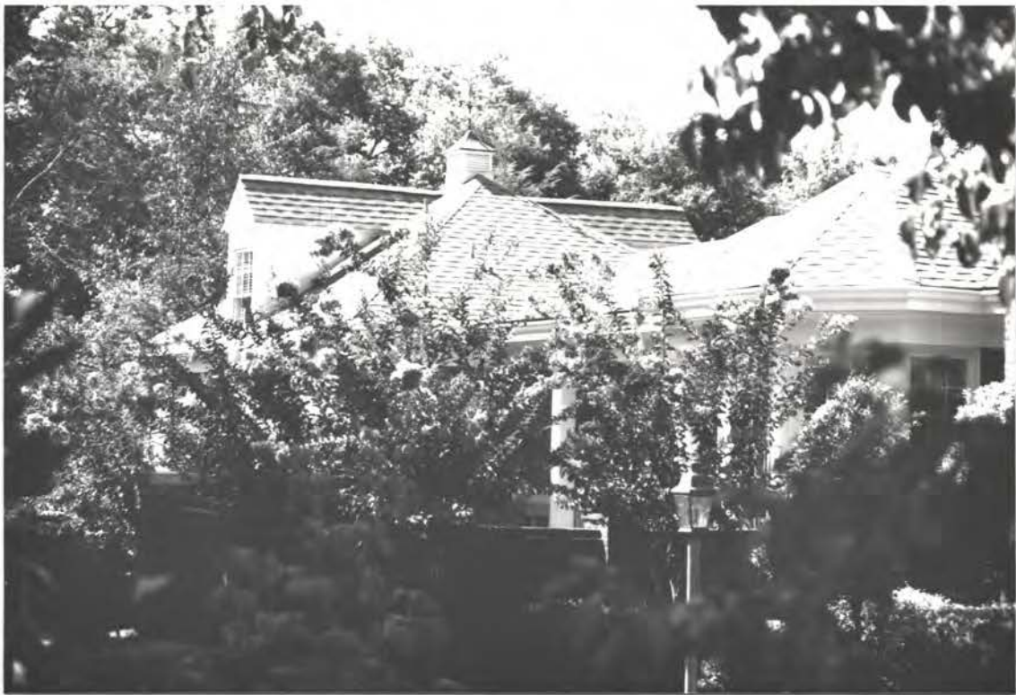
poor execution by contractor - dormers not as detailed, framing revised in a structurally risky way, etc. (Burl Chandler, contractor)
