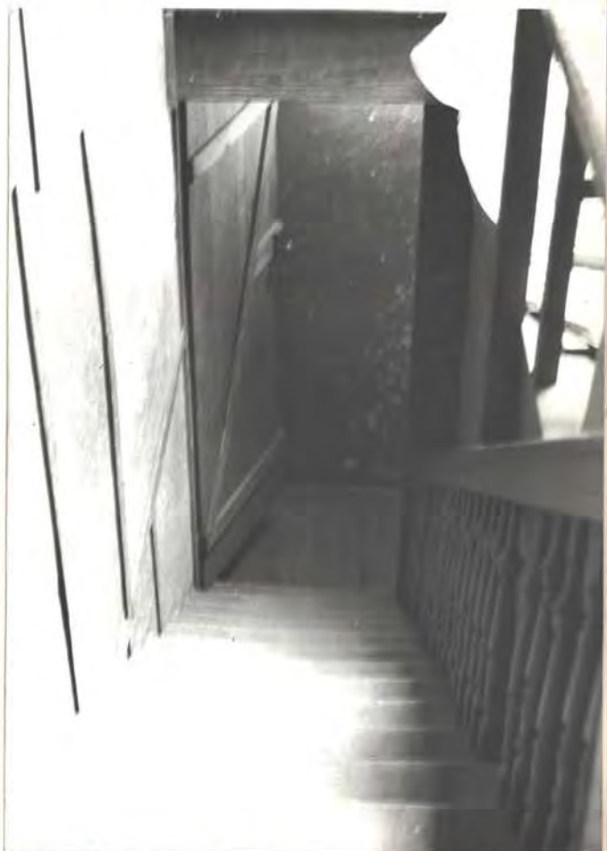
Stair from east 2nd fl. down to east main fl. (see photo at left)
