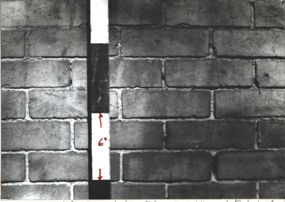
East wall (exposed to SE) = "NO. 1" quality bricks (S. front = same) All-running bond
