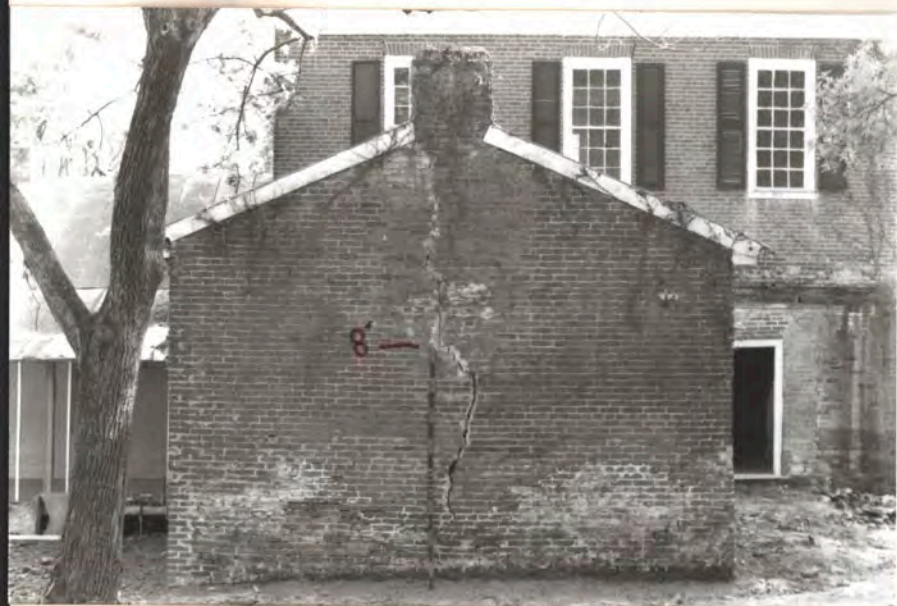
Fed Ell Add. - bowed + cracked wall
