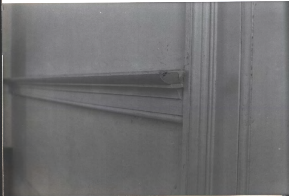
Chair rail at 2nd fl. hall, w. wall → A DOOR ↗ (end has been cut off 45° later)
