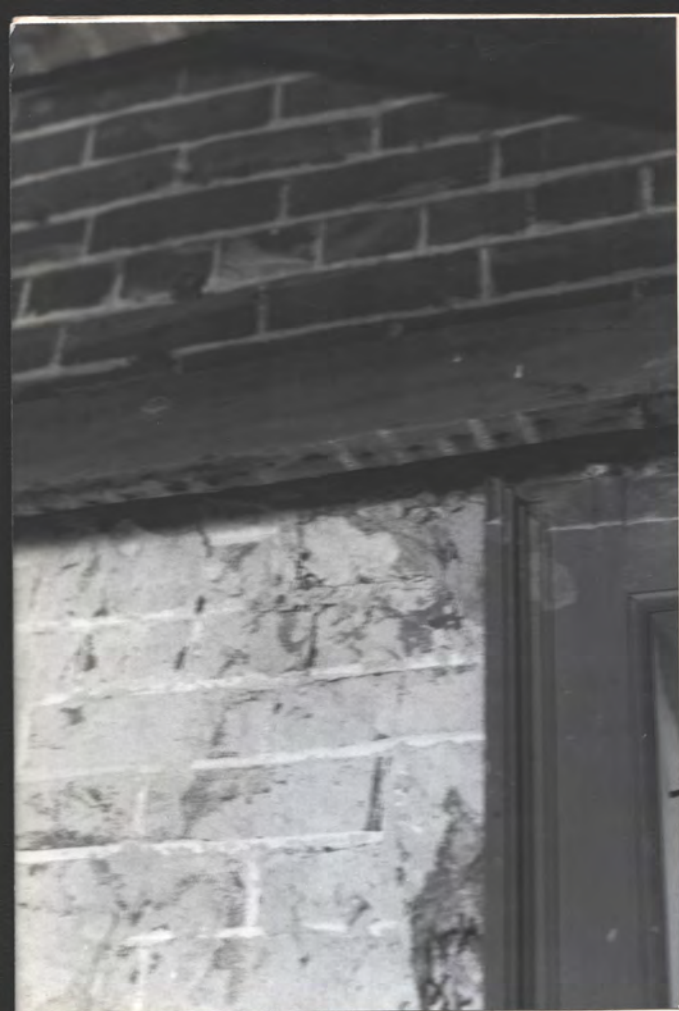
white paint stripe "penciling" at brick joints
