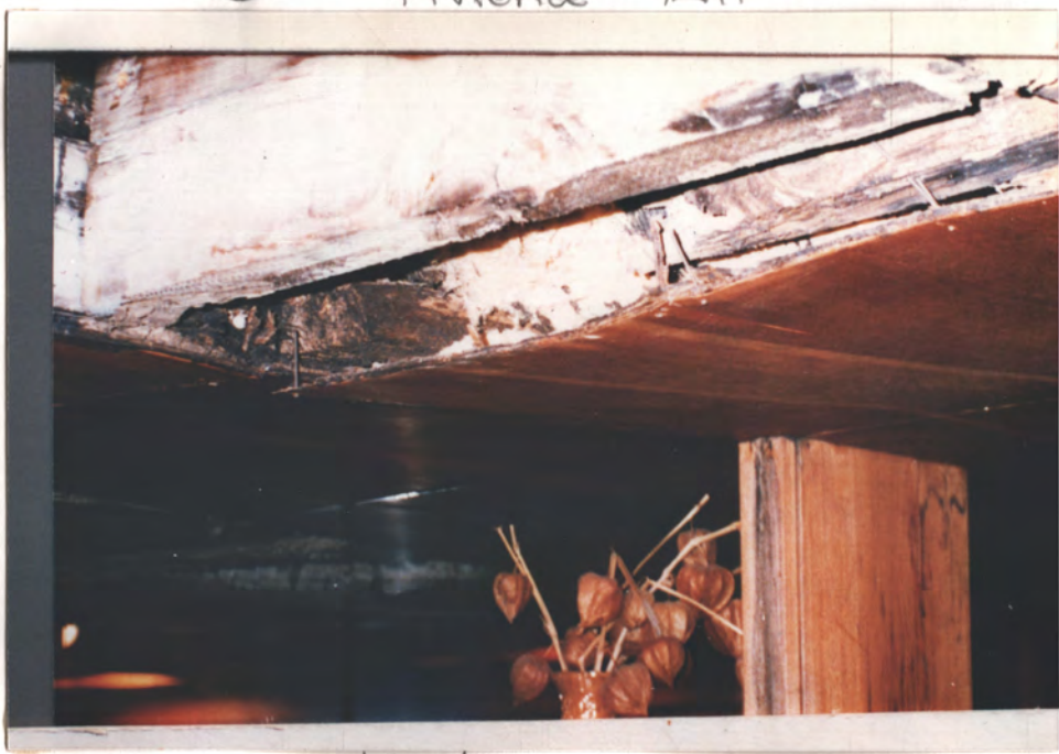
NE Wing, Bkfst roof rot
