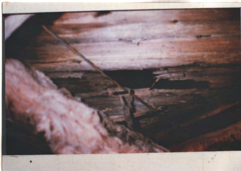
Bkfst — roof rot
