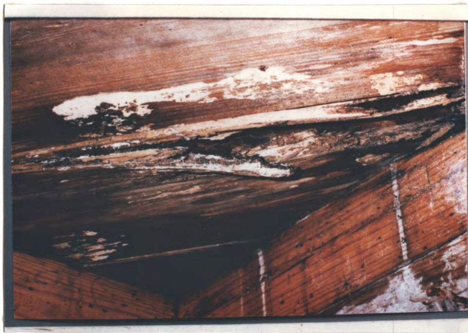
Bkfst - roof decks rot
