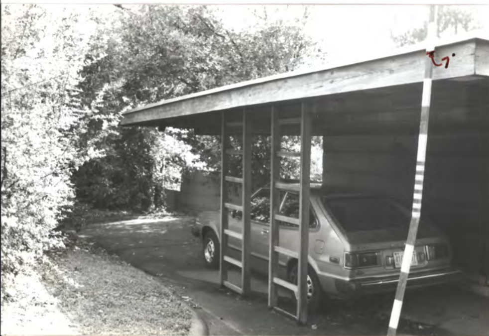
1948 erect carport (trellis added later, c. 1968, when roof deflected) - per Mrs. R.
