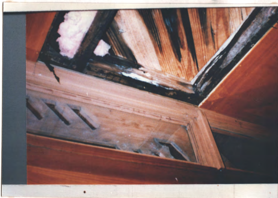
E. Hall, rot & termites
