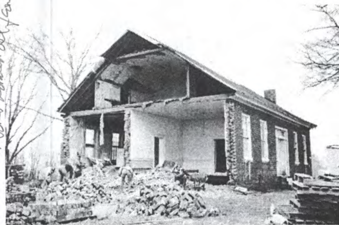
Emergency cleanup crews dispatched by B.H. Craig Construction, Co. after the Dec. 27 collapse. The c.1850 Koger House once had dormer windows.
