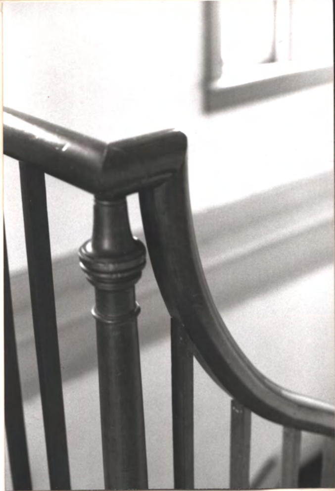
2nd fl. railing → W
