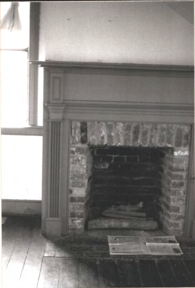
AN 2nd fl. front room mantel. "Surround" should be plastered. Handls pattern not correct
