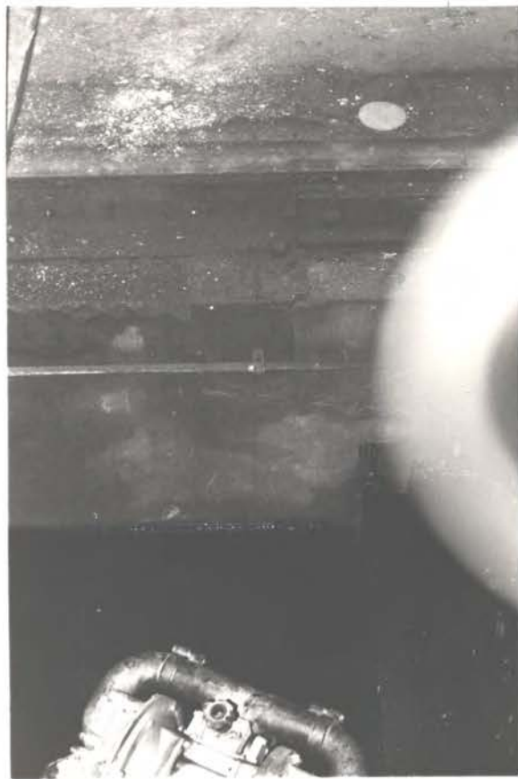
↑ work pit (flooded)
