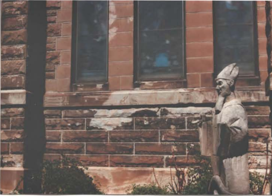
1 Stone spalls & patches, Rising damp deterring.
