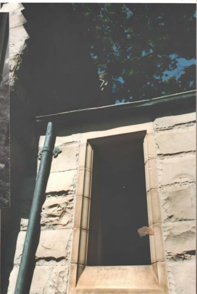
SW. Steps - bent copper gutter Not 4 10
