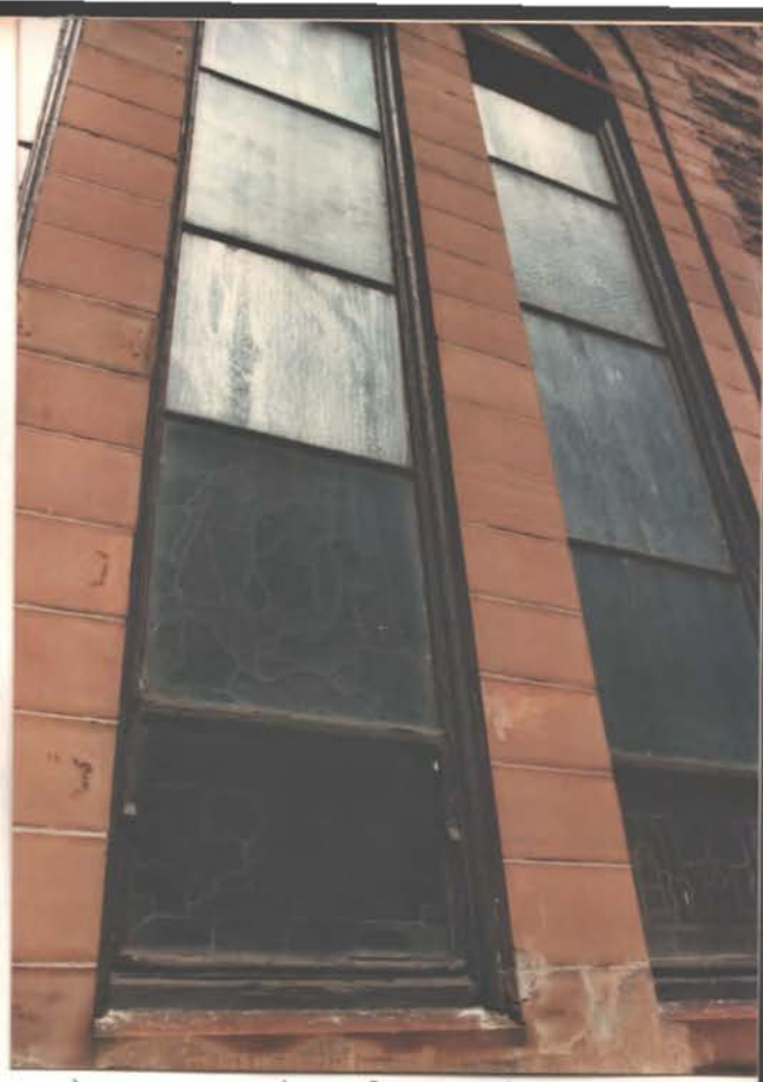
S. Wall at Garden Ribbed protective glass (in steel sash set in orig. wood frames)
