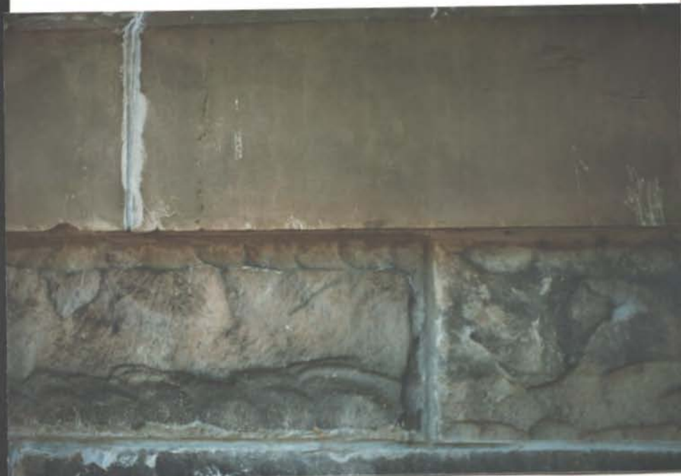
apparent portland cem. re-pointing 1 \frac{1}{2} N
