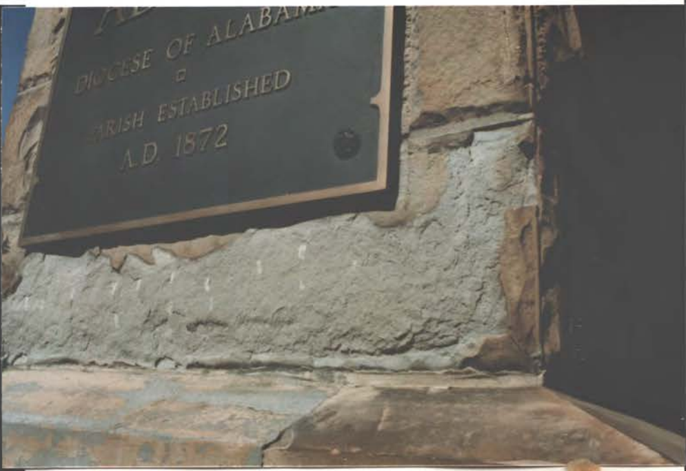
↖ Cement "rebuilding" of stone parts + spalls 3 — West front
