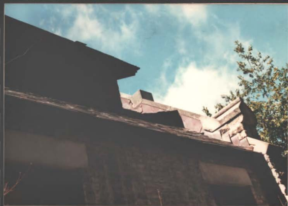
1 → N East Wall of Clingman Commons (no gutter: runoff soiling + damage)
