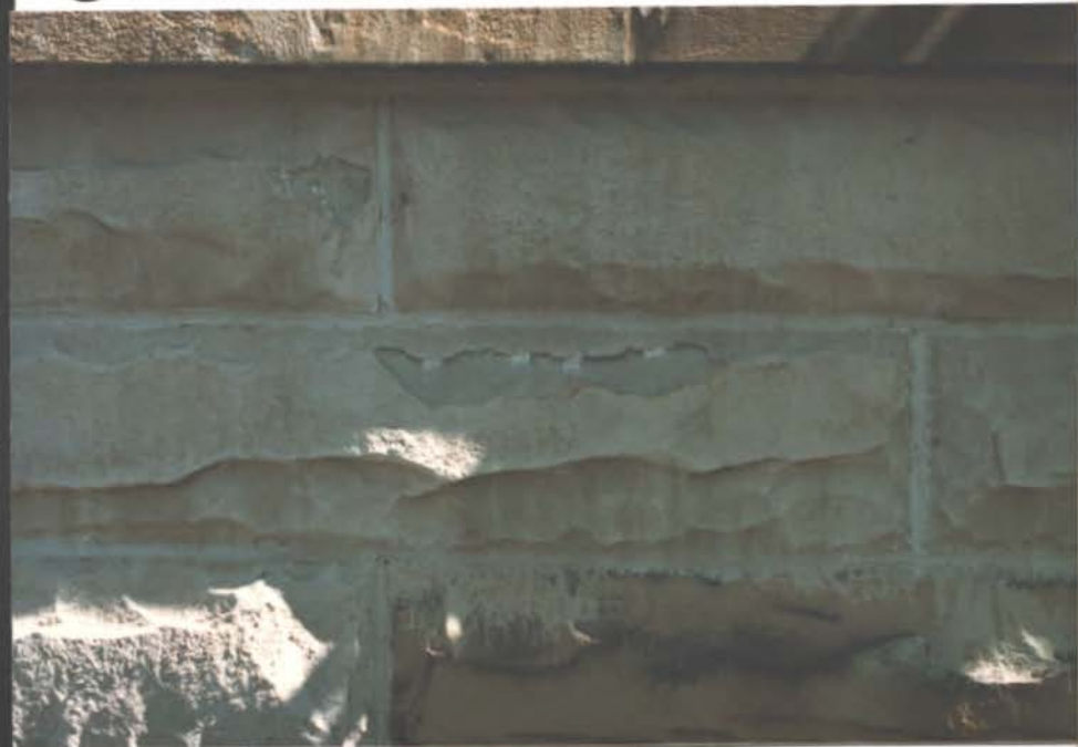
3 Spalled & coated sandstone \frac{1}{2} N
