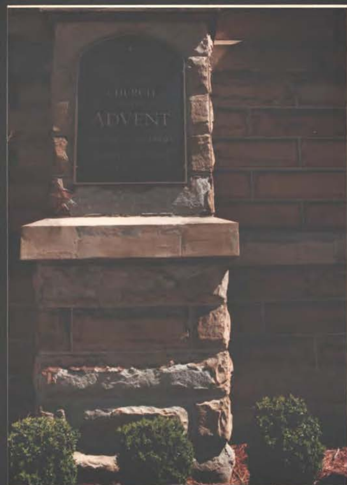
Bell tower N.W. Corner 1 N+ Rising damp deterioration
