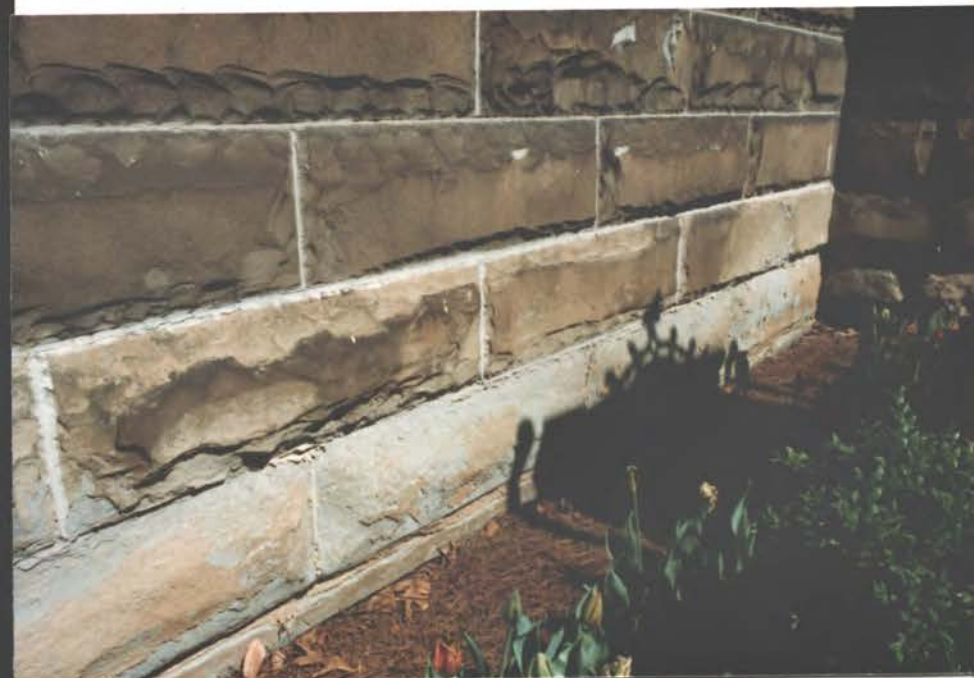
Not ↑ West front, S. part. Low grade traps water against stone. ↓ Spalls & rising damp deterioration
