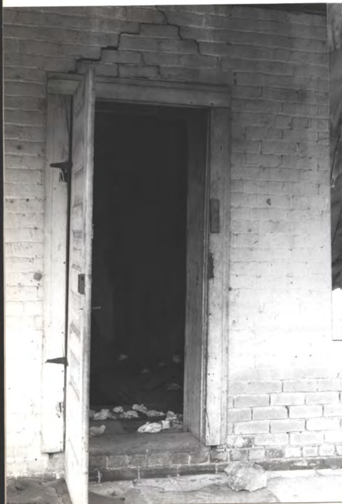
WEST 20TH C. DOOR, APPEARS ADDED
