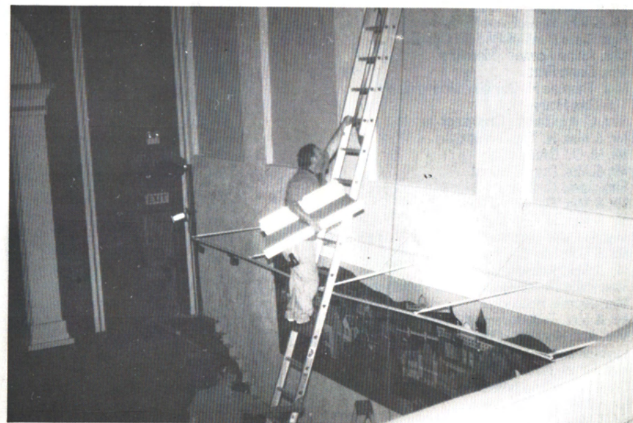
John Hegwood climbed forty-five feet in order to install gold caps to wall panels in the theatre.
