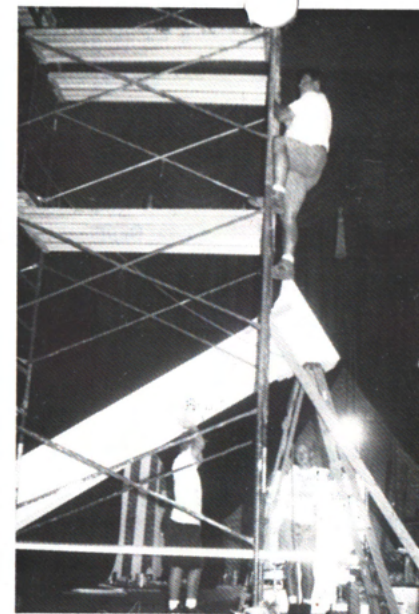
Jonathan Harris (top) climbed the scaffold in preparation to anchor one of the heavy columns with the help of two workers on the stage floor.
