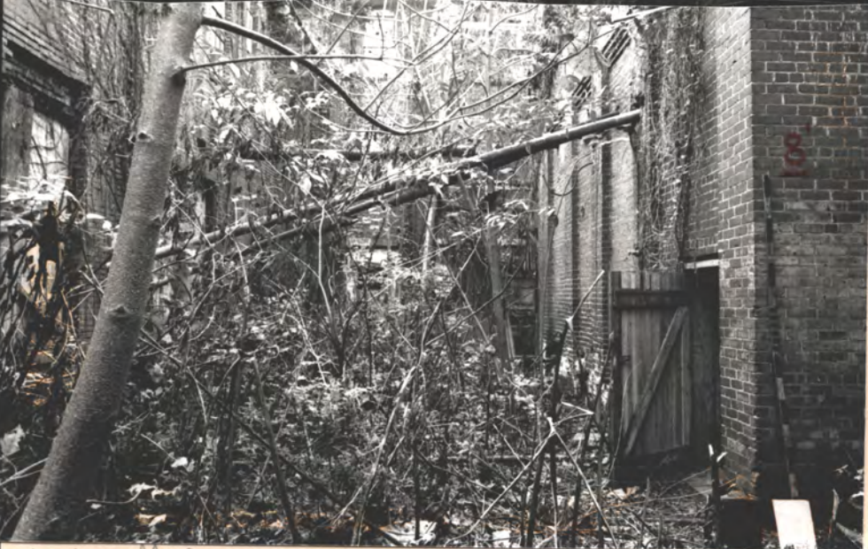
W. Wall of N. Cent. Bldg E. Wall of Boiler Hse (C)
