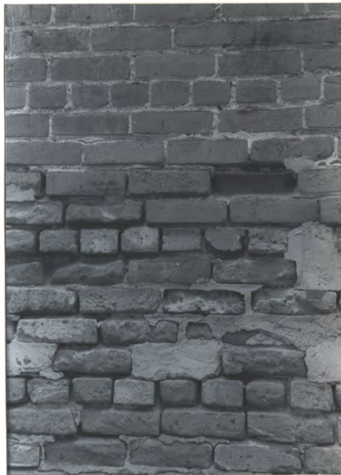
Soft deteriorated local brick on N. wall
