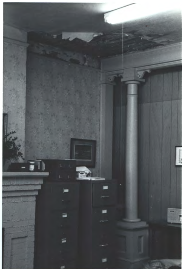
Fed. front center rm. Beam + Col. = Vic. Mantel = c. 1920's Bungalow style. Note Fed. split-both at ceil.
