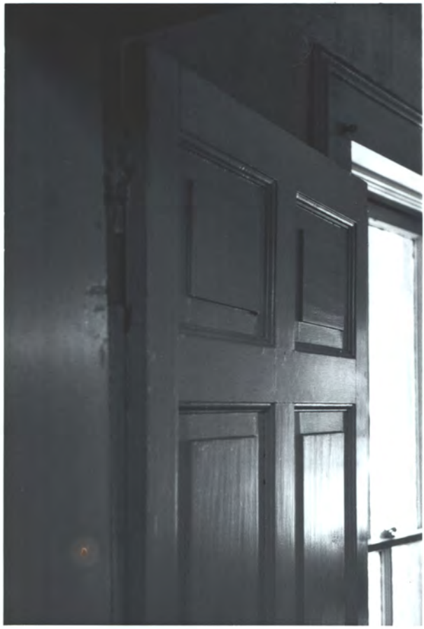
Fed. 6-pnl. hand-planed mortised & tenoned & pegged door. Front center rm. to left front rm. Note above on 1.
