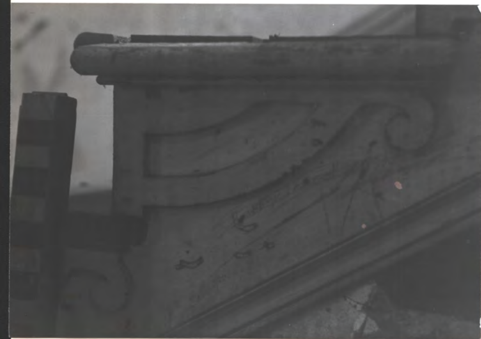
MAIN STAIR (BALUSTRADE GONE)
