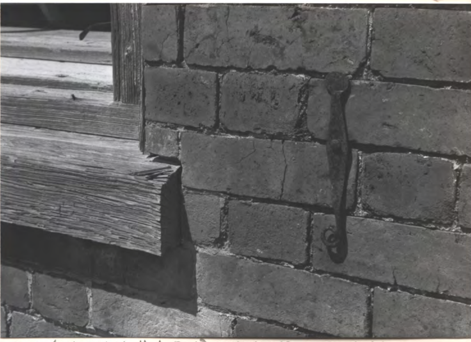
SHUTTER - DOG (MATCHES H.A.B.S.) - ONLY ONE REMAINING 2ND FL. S. WALL, W. WINDOW. HAS BEEN FLATTENED - SEE H.A.B.S.)
