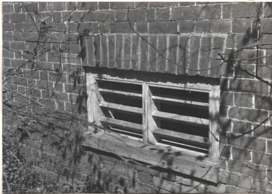
WEST WALL ENDN. VENT
