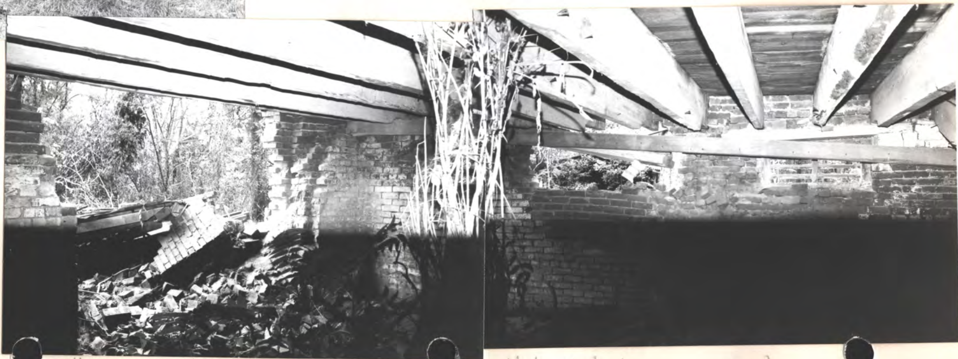
collapsed pent A
