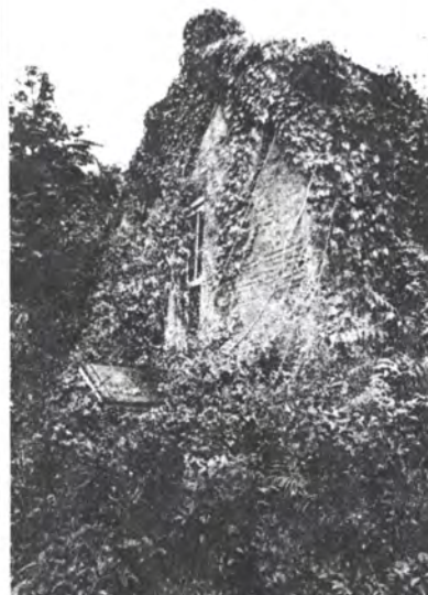
Although derelict, the c.1828 Belle Mont house was an attractive candidate for restoration because it had never been remodelled.
