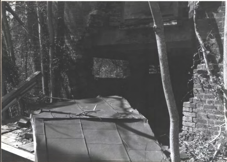
PENT ROOF COLLAPSED (SEE H.A.B.S.)
