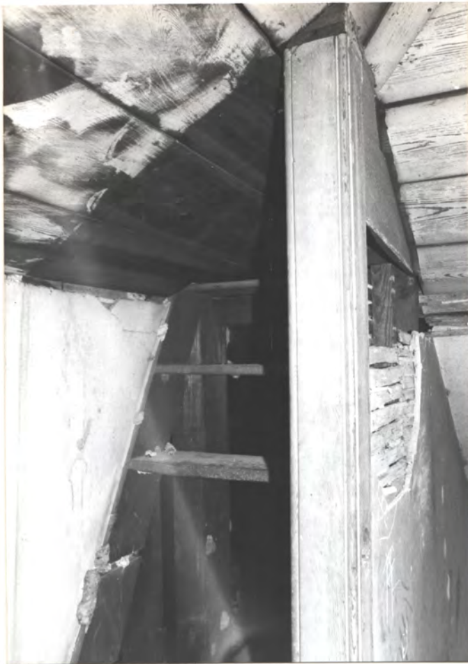
Stairs up to former roof deck on top of 2nd fl. partition roof
