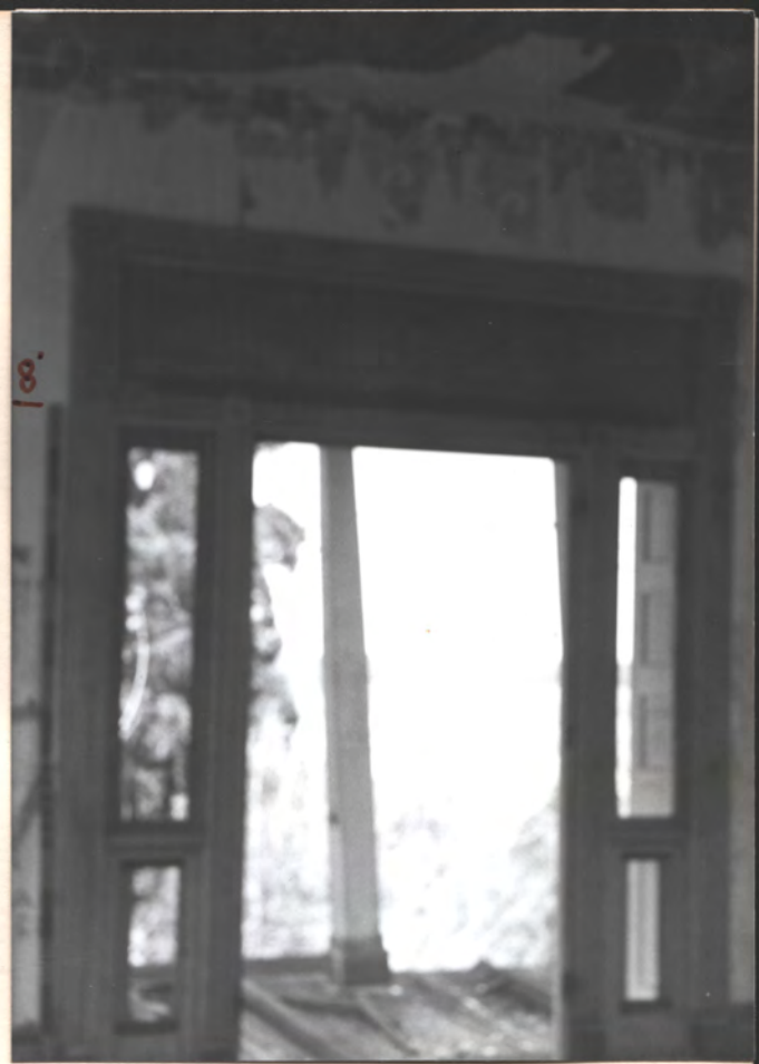
2ND FL. N. DOOR TO UPPER TIER OF PORTICO (ENTASIS ON COLS., SOLID WD) MUNTINS & LOWER PNLs KICKED OUT
