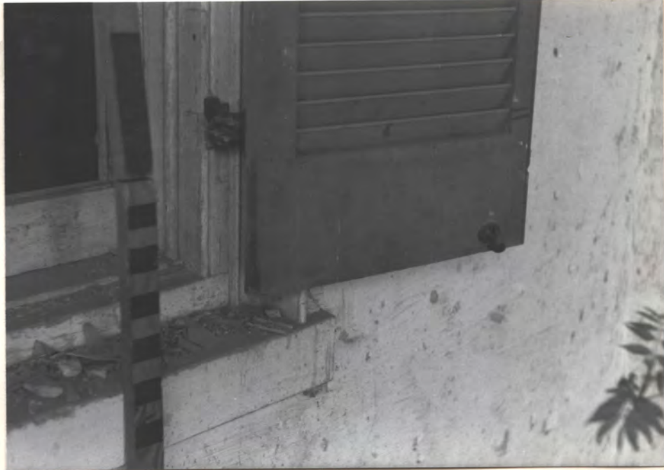
W. WALL PATIO, N. SASH. CAST IRON HINGE LATER , SEE HINGE-PATCH ABOVE IT, & PG. 13 HINGE
