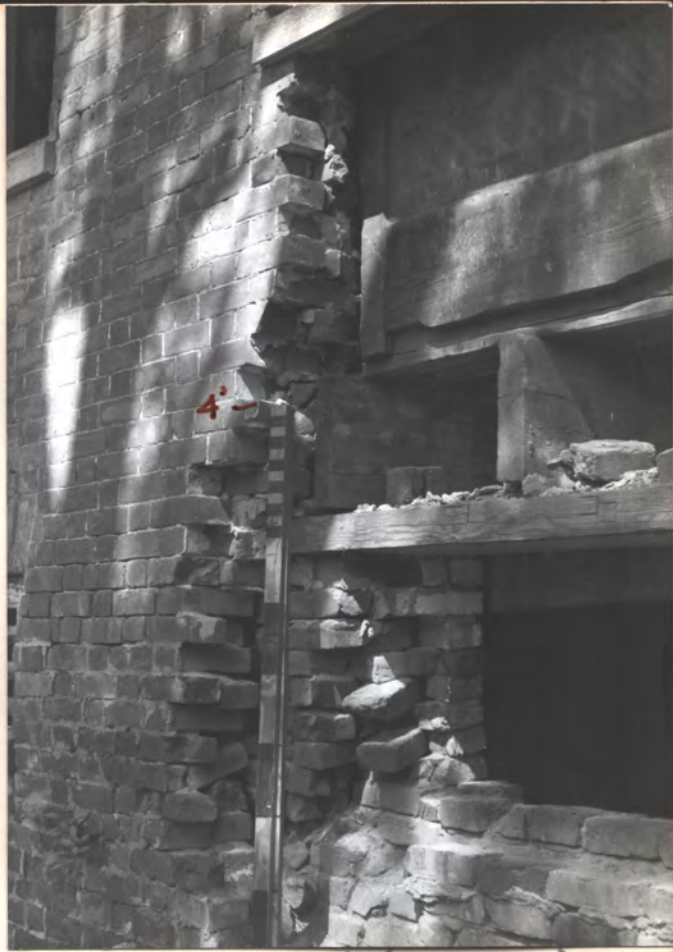
W. SASH IS ABOVE (S.W. WING) VENT WAS HERE FL. JOISTS + FL. IS ABOVE
