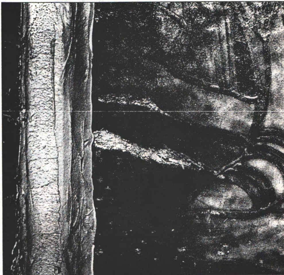
The white smudge at the left center of this panel used to be a lead came. When the protective glazing was installed, it was placed flush against the stained glass. Since the stained glass could not be sealed, water vapor infiltrated the cavity. In cold weather, it condensed on the lead and, in a period of less than ten years, turned the lead to powder.
