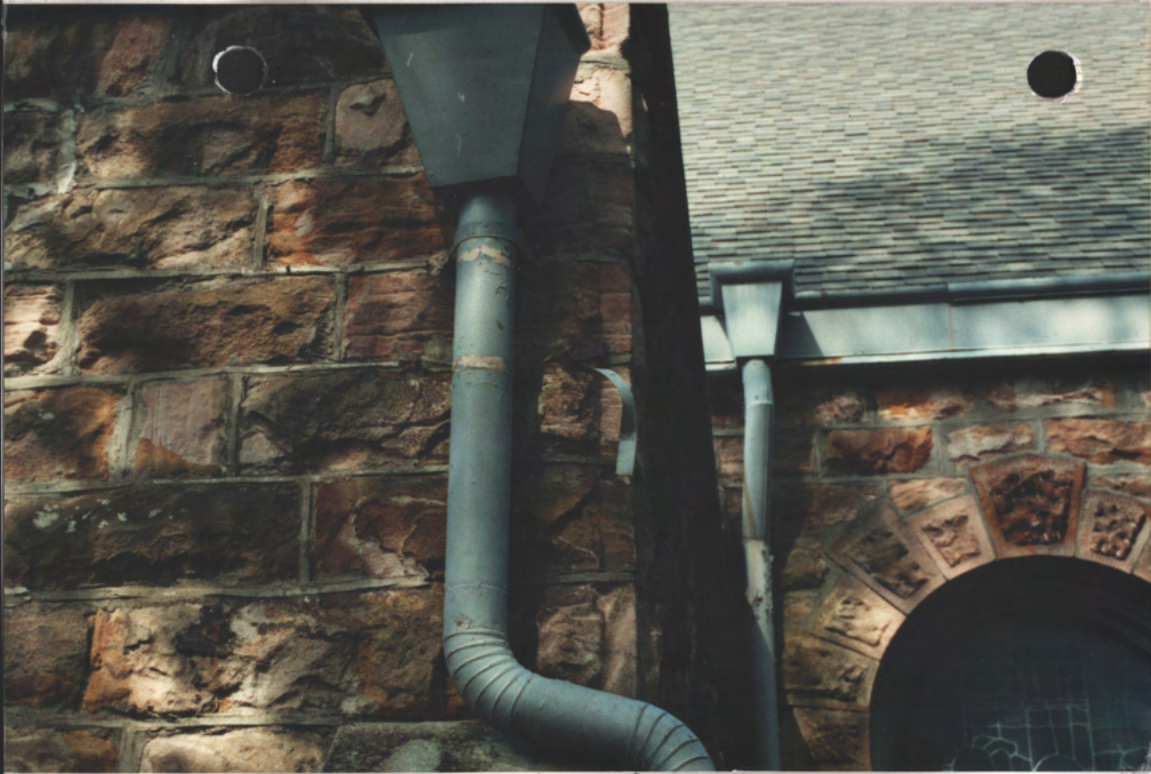
Spilled stone → → N.E. Corner of S.E. Ambulatory
