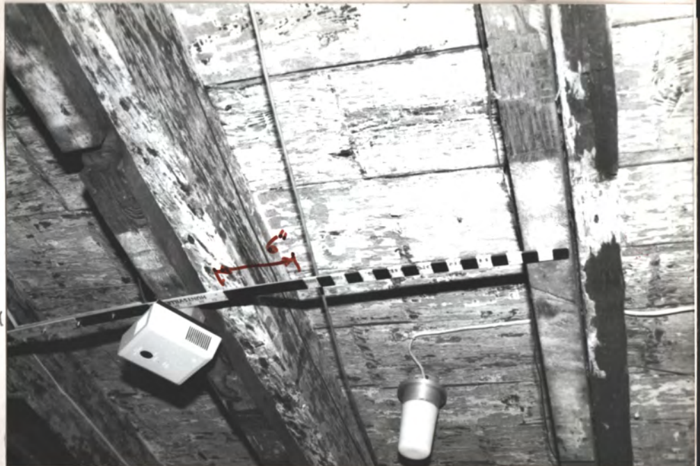
Note - the very wide, thick pine pl. is REUSED from another bldg. - (WIKI? 1926 or 1960s?) The hatchet leveling - places don't align with these joints
