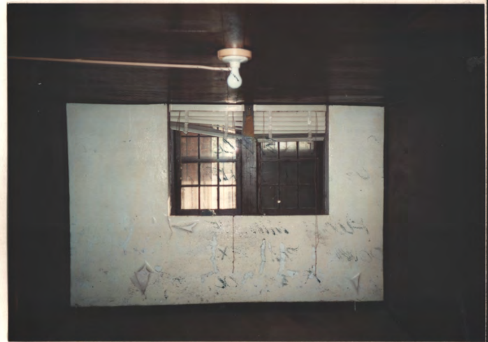
around the windows are under front story level 1
