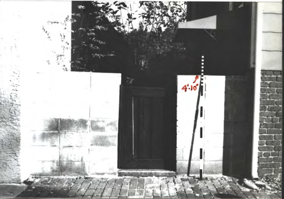
Mod. conc. blk. wall at west yard, at E. Bay St. 9N
