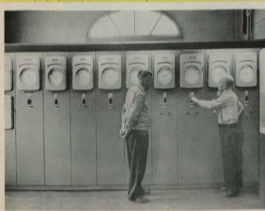
James S. Wall (left), water superintendent, and T. J. Hicks, pump operator, at central control panel.
