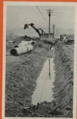
More sewer lines are laid as city moves to service all areas.
