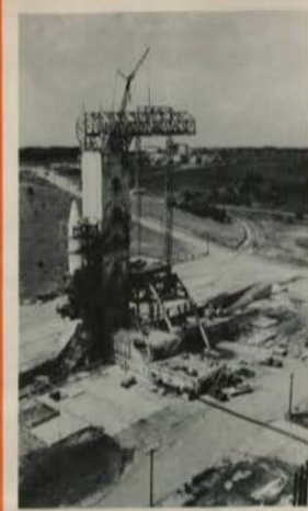
The test stand at ABMA, showing modifications to handle the mighty Saturn booster.
