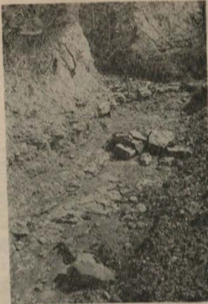
Plate 12-A.—Contact (shown by geologic pick) between basal sandstone bed of Chattanooga shale and underlying shales of the Red Mountain formation in road cut 2 miles west of Plevna, Ala.
