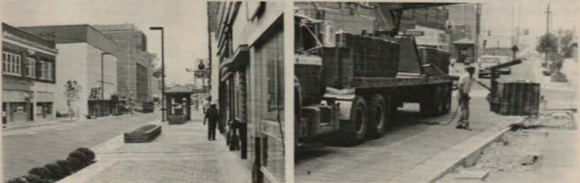
Above, left looking south from the corner of Jefferson and Holmes one views the nearly completed street. Kiosk lacks phone and news rack. Central city parking facility is on left beyond sterchis. Above, right, looking north just outside parking facility, contractor offloads sidewalk bricks as traffic moves around and through construction. At press time this work was virtually complete.
