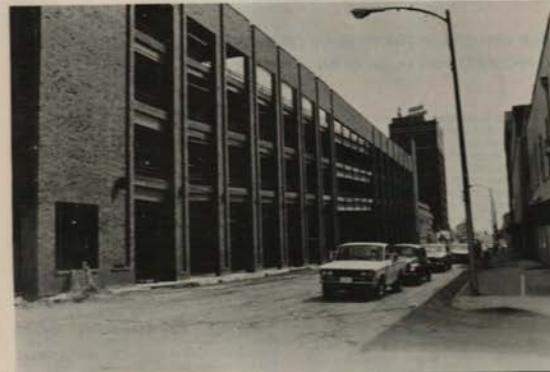
Downtown parking facility nears completion, as street work progresses on Clinton Avenue between Washington and Jefferson.
