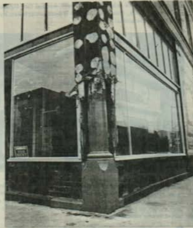
Figure 6. Storefronts of the 1940's, 50's, and 60's were frequently installed by attaching studs or a metal grid over an early front and applying new covering materials. If the existing storefront is a relatively recent addition with little or no architectural merit, begin by removing the covering materials in several places as was done here. If this preliminary investigation reveals evidence of an earlier front, such as this cast-iron column, carefully remove the later materials to assess the overall condition of the historic storefront. The black mastic visible on the lower masonry panels was used for installing pigmented structural glass. Some attachment methods for modern facings, such as mastic or metal lath, may have seriously damaged the original fabric of the building, and this must be taken into account in the rehabilitation process. Photo: Bob Dunn
