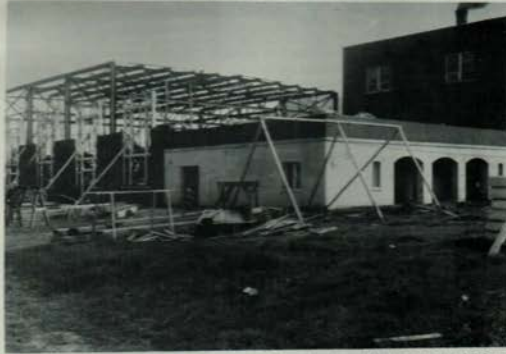
This view shows the construction of the school auditorium and additional rooms in 1928. Expansion of Joe Bradley School was undertaken several times by Merrimack Mfg Co., after they built the first section in 1919. (Photograph Property of Huntsville Parkers)
